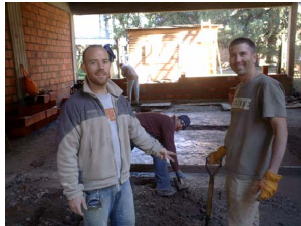
Ryan Moore and fellow Builders International Missionary Sam Fenton, at work on the Rio de la Plata Bible Institute.
